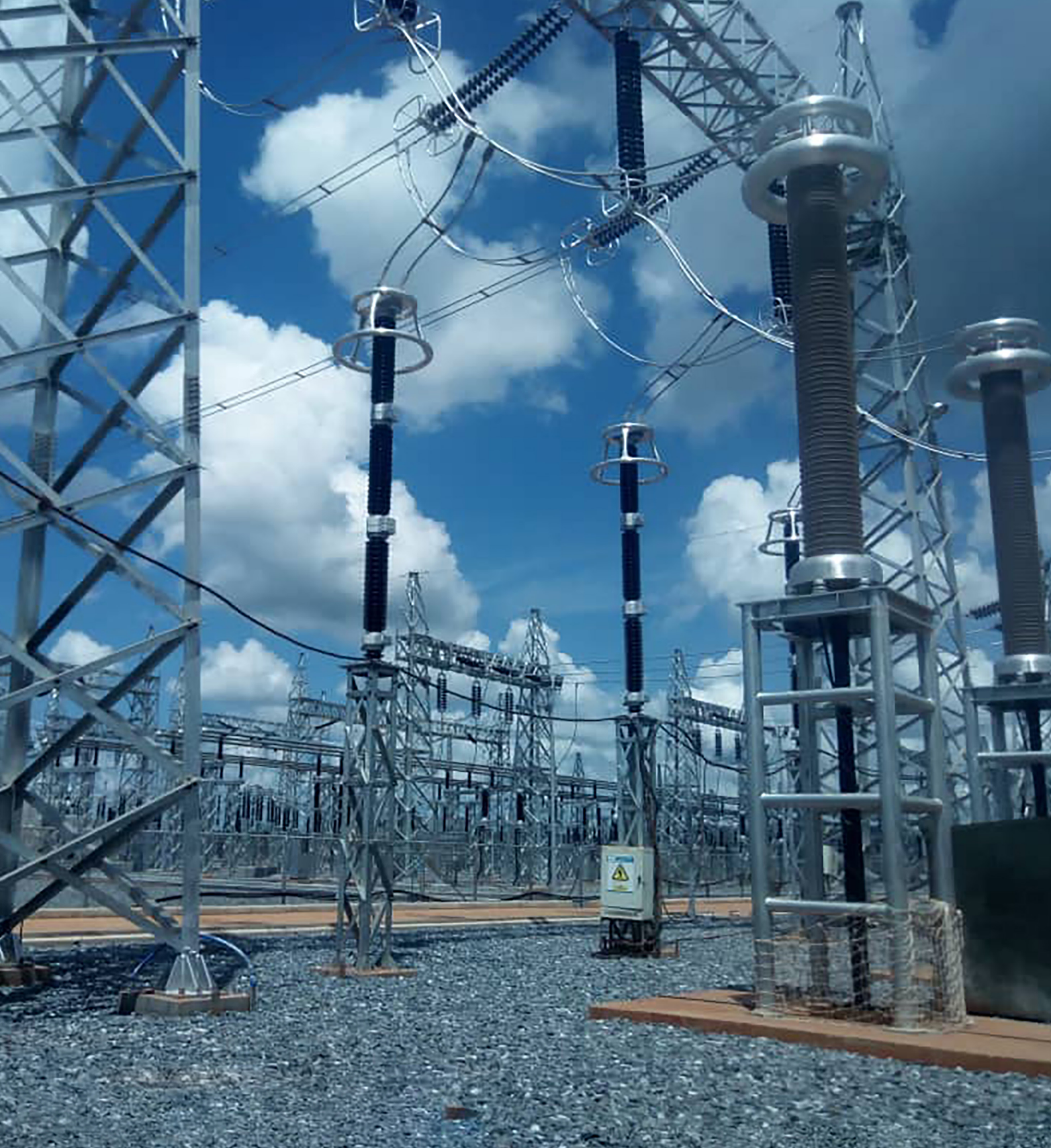
The 400kv Karuma Sub Station
