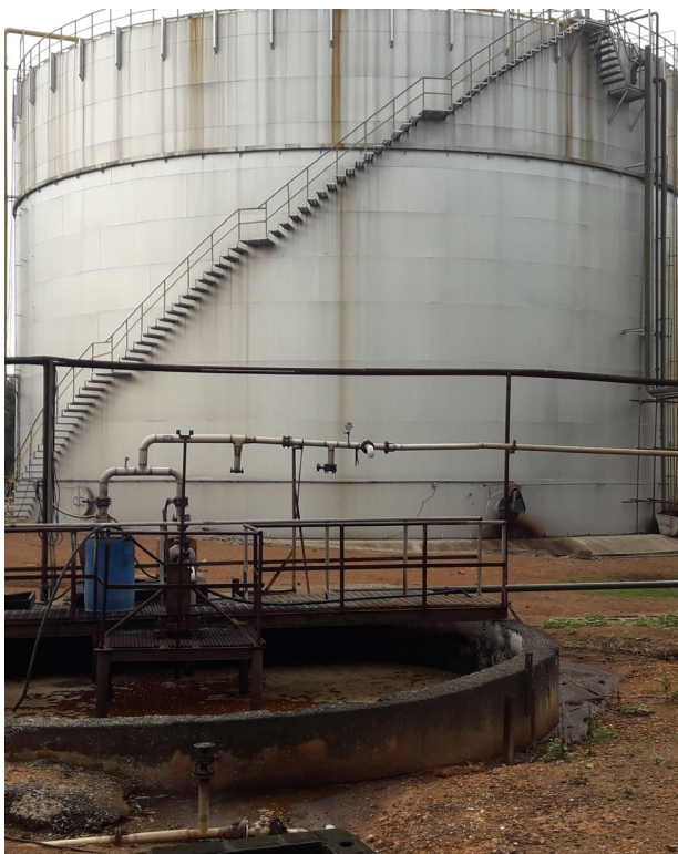
Biogas Plant generating Methane Gas used for firing Boilers in a distillery
